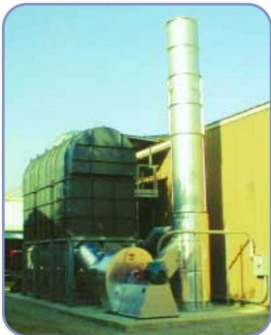
Eurocad RTO (regenerative thermal oxidizer) installed at EP Graphics in Berne, Indiana.
