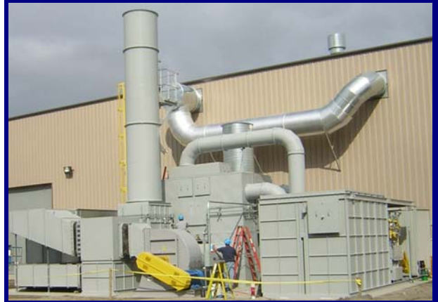
2009 installation of a 40,000 SCFM Concentrator with RTO system with integrated building make up air heat recovery for a surface coating operation in North Dakota.
