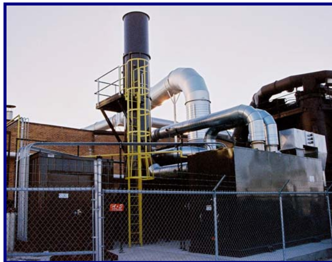
30,000 SCFM Concentrator and Catalytic Oxidizer System installed at an Illinois facility.
