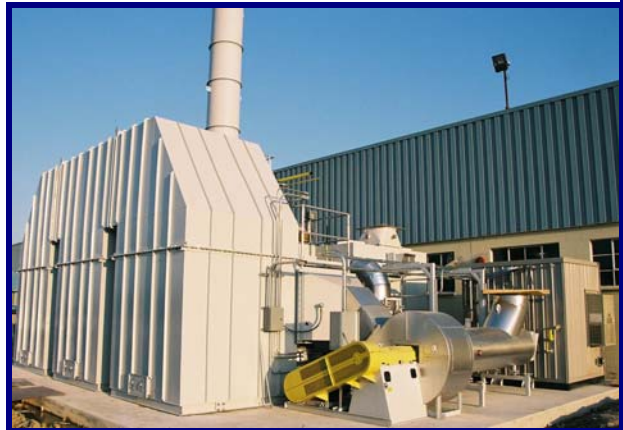
A Hybrid 22,000 SCFM Concentrator and 12,000 SCFM RTO System installed at a Michigan facility.
