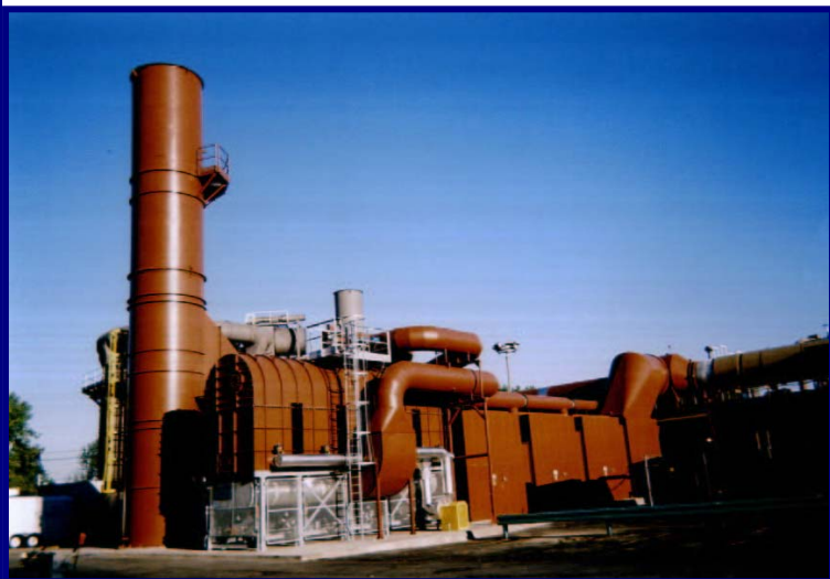
250,000 SCFM Concentrator and RTO System installed at an Ohio facility.
