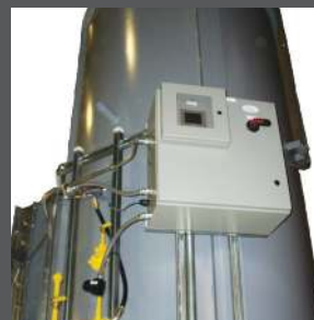
Lower Section of Flare with Control Panel
